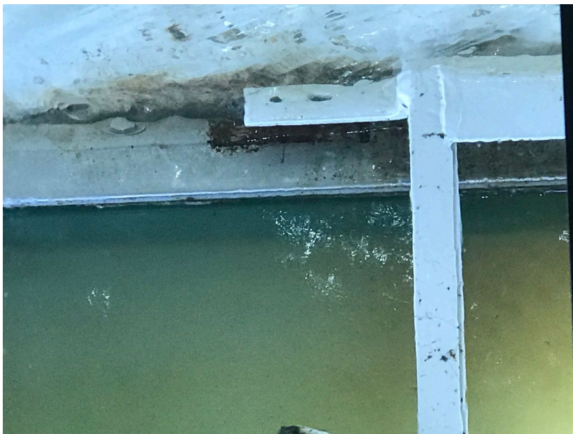
Photo 2. Close up of disconnected backboard bracket.
