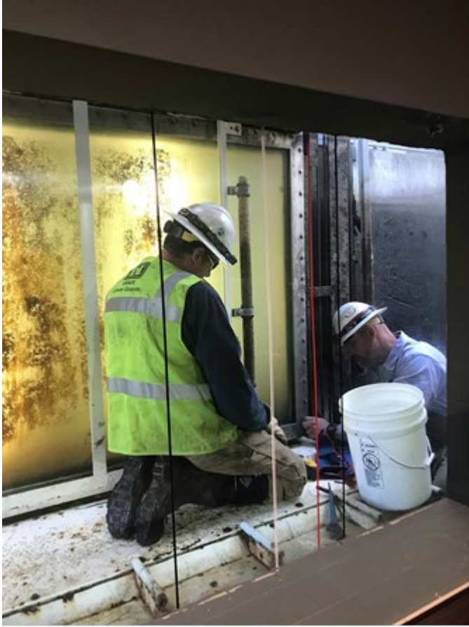
Photo 1. LWG fish ladder PH mechanical crew repairing the fish count window backboard frame.
